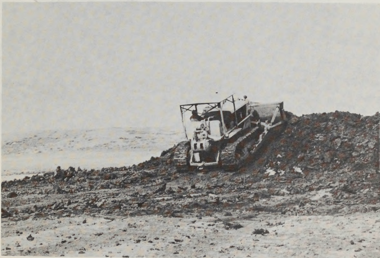
Illustration 3. Dirt mound islands can be push up with a bulldozer during periods of low-water levels in existing reservoirs. Islands are most easily accomplished during reservoir construction with similiar equipment.
